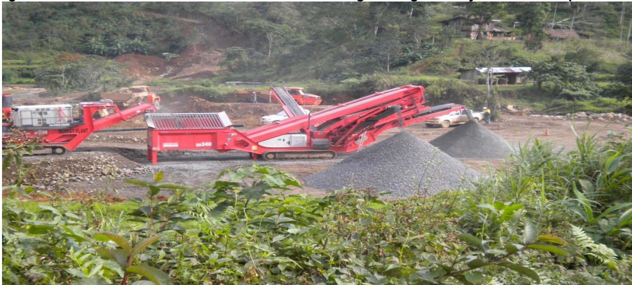
Figure 1: Crusher for construction material for the Tailings Storage Facility on site at Didipio
